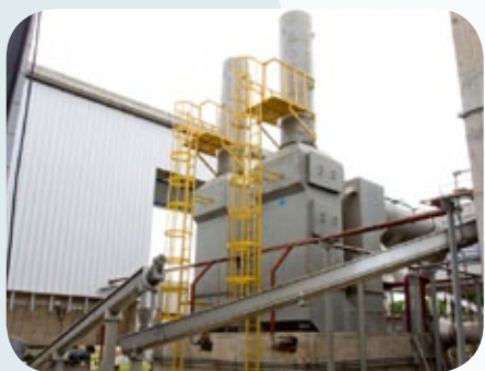
Gases washer (scrubber)
