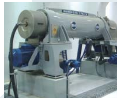
Impianto municipale trattamento acque reflue - Municipal waste water treatment plant - Station d'épuration des eaux usées ménagères
