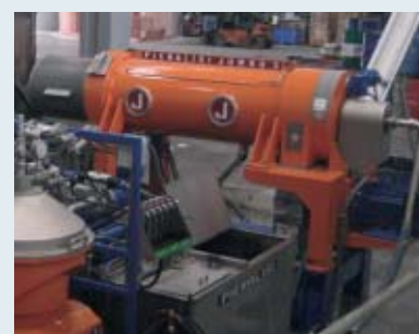
Trattamento oli slop - Treatment of slop-oils - Traitement des slops pétroliers
